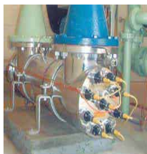
Figure 5: Wedeco – Ideal Horizons UV reactor installed at the Norfolk Spruce Road Well facility.
