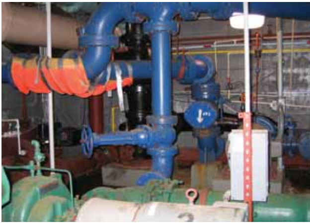
Figure 1: Illustration of the tight quarters in a Small Water System in New Hampshire (photo courtesy of Cynthia Klevens, New Hampshire Department of Environmental Services).
